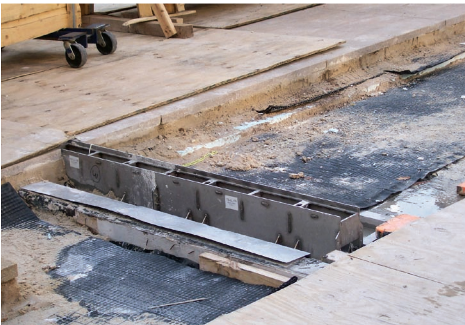
JES Plumbing used pre-assembled, fabricated trench drains custom-made by Jay R. Smith Mfg. Co. for the renovation of New York's esteemed Lincoln Center.
