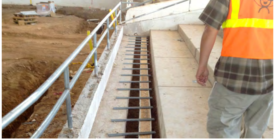
By installing the Enviro-Flo drain from Jay R. Smith Mfg. Co. in Scottsdale's Equestrian Center, staff can hose down the seating area after events without worrying about the water flowing into the arena's dirt floor. The Enviro-Flo was easier to install than standard floor drains, saving time and money.
