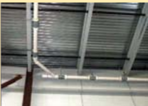
The horizontal manifolds in a siphonic roof drain system installation.
