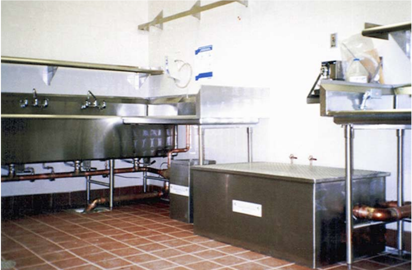
The Remediator® Grease Treatment System Fig. No. 8970 installed on kitchen floor
