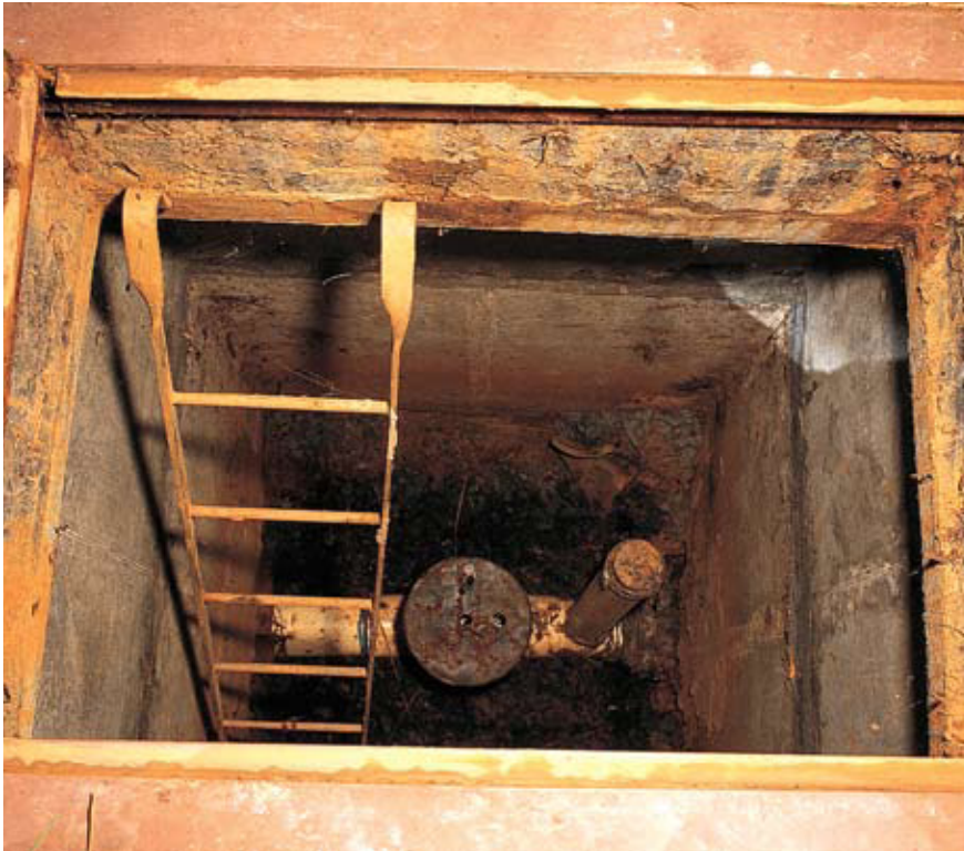
View looking into pit of Flood-Gate® & cleanout.
